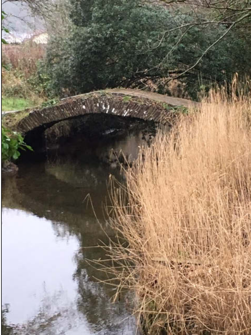
Photo taken in 2018 after CVCP had restored the bridge with funding from the Landfill Communities Fund received through ENTRUST.
